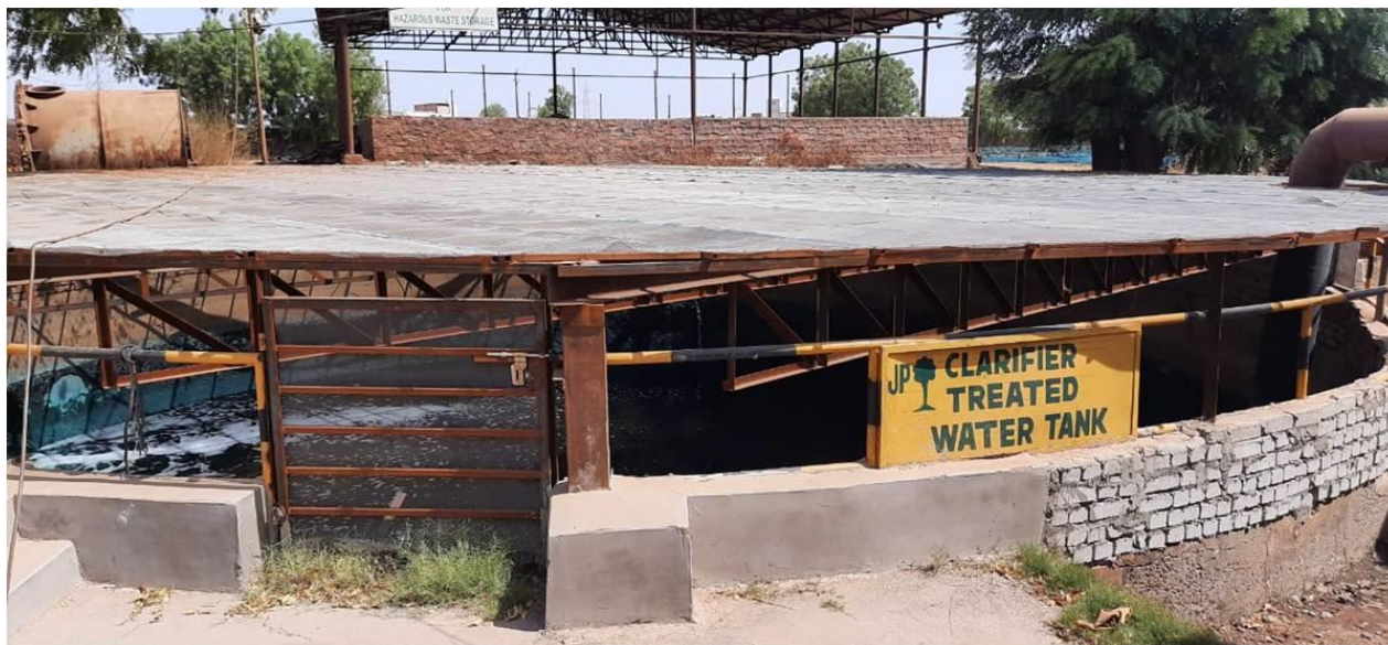
Clarified Treated Water Tank
