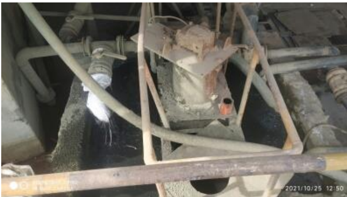
Primary Sludge Sump
