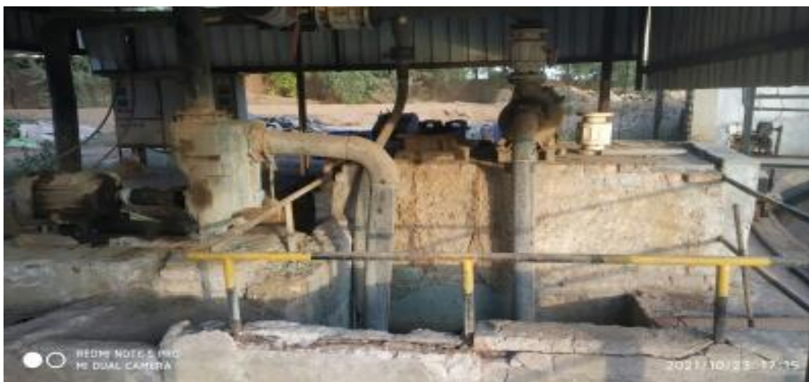
Secondary Sludge Sump
